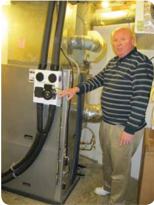
David points out that the pump for the geothermal HVAC system does not need to be very large or powerful.
