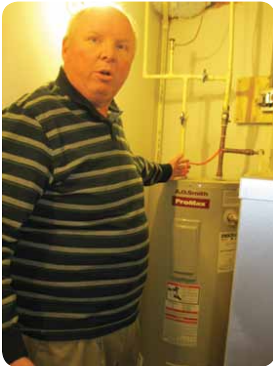
David demonstrates how their geothermal HVAC system preheats water for their hot water heater.
